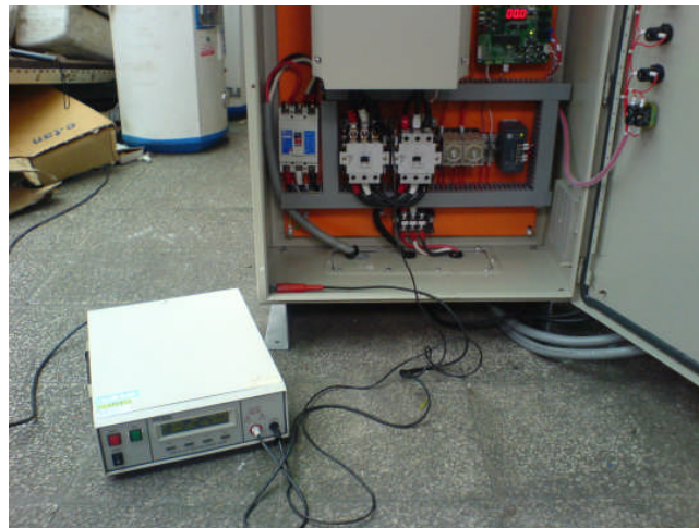
Insulation resistance test
