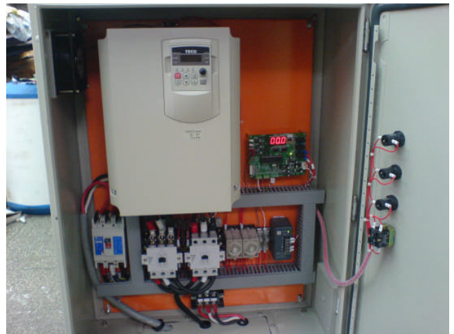
Control panel of machine
